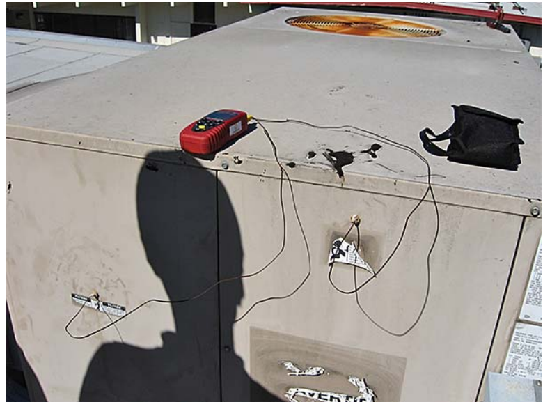
Figure 3. Showing the digital thermometer reading temperatures before and after the evaporator
