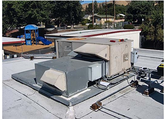
Figure 1. View of rooftop unit with school playground in background
